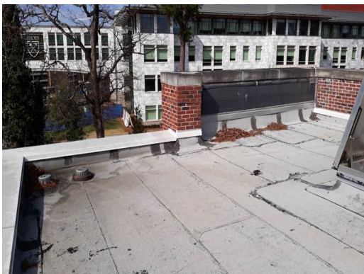
Debris Throughout Roof And At Roof Drains Need To Be Cleaned
