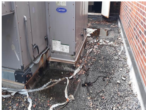
Built-Up Roofing Over Original Modified Bitumen Roofing Are Beyond Useful Life And Need To Be Replaced
