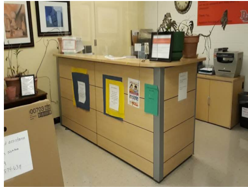
Administrative Office Counter Is Non-ADA Compliant. Counter Needs To Be Retrofitted To Make ADA Compliant
