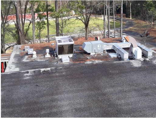
Built-Up Roofing Is Beyond Useful Life And Needs Replacement
