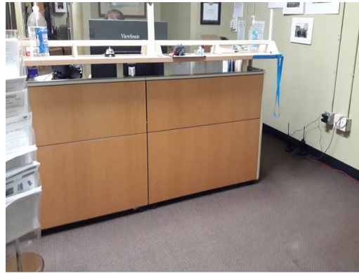
Main Office Reception Counter Is Non-ADA Compliant And Needs Retrofit To Make ADA Compliant
